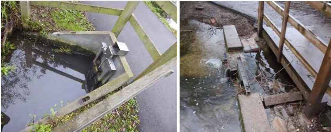
Sluices at inflow to Batchworth Lake and outflow from Bury Lake.
